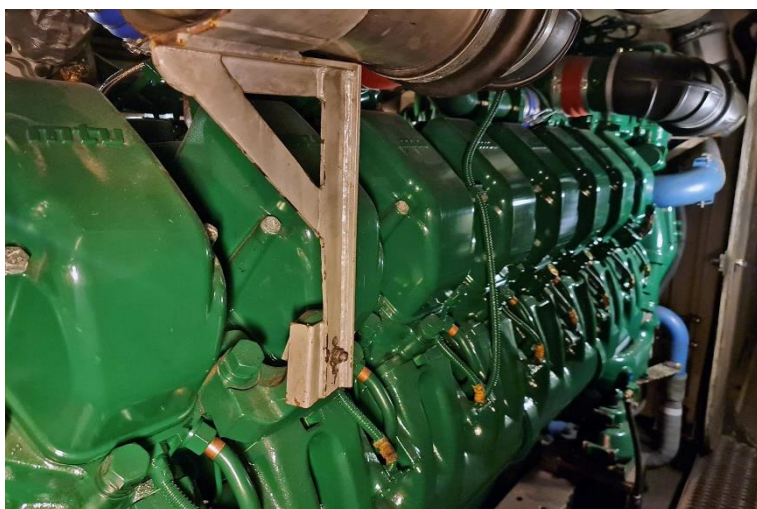
MTU Power Unit
